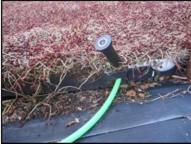
This Live Roof tray system shows a 6" pop up spray without support. Each time the irrigation is turned on the head will continue to loosen, over spraying irrigation, wasting water and irrigating areas NOT intended for water.
