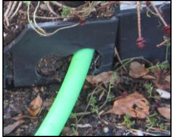
Live Roof tray system showing signs of alterations to account for irrigation line compromising the integrity of the tray.
