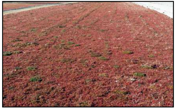
Green Living Roof (Winter)
