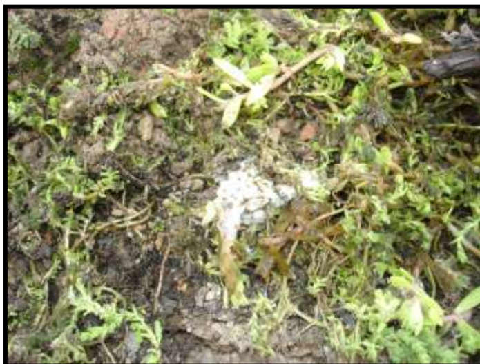
Fungus developed because the panels were left stacked too long.
